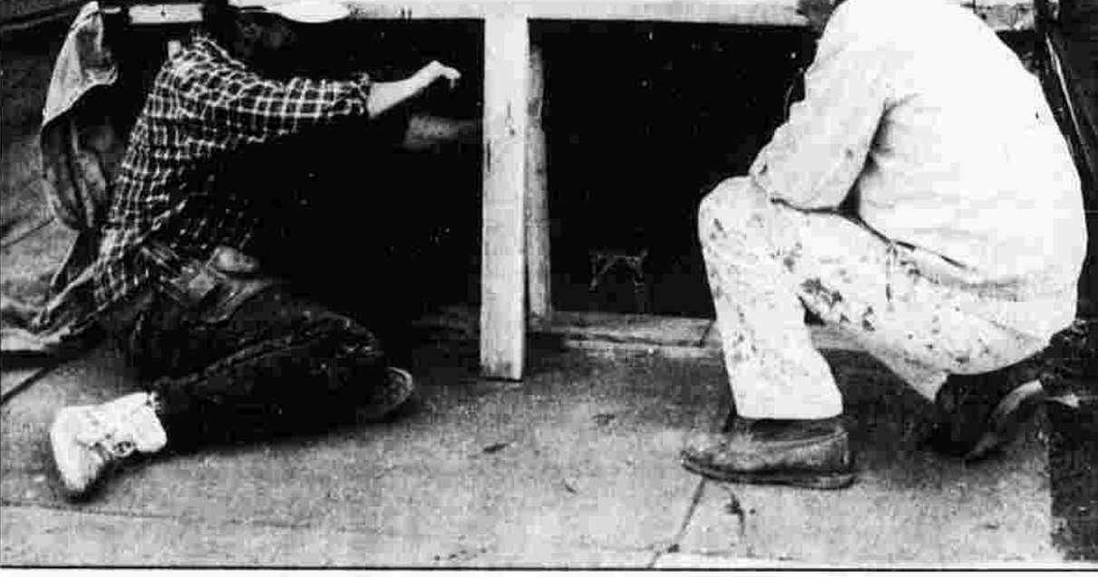
SUPPORTING CAST — Dwight Petersen, left, and Lawrence Gavello, both of Manchester, work on supports Thursday for work at the Bissell Candy Co., 18 Bissell St.
